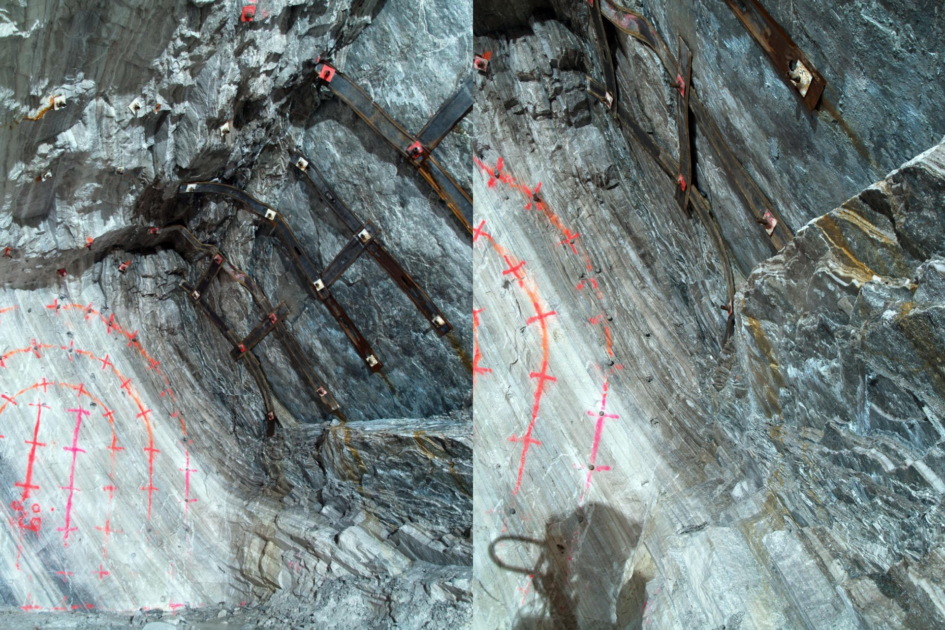
Fault along Right Wall - Station 3+23
