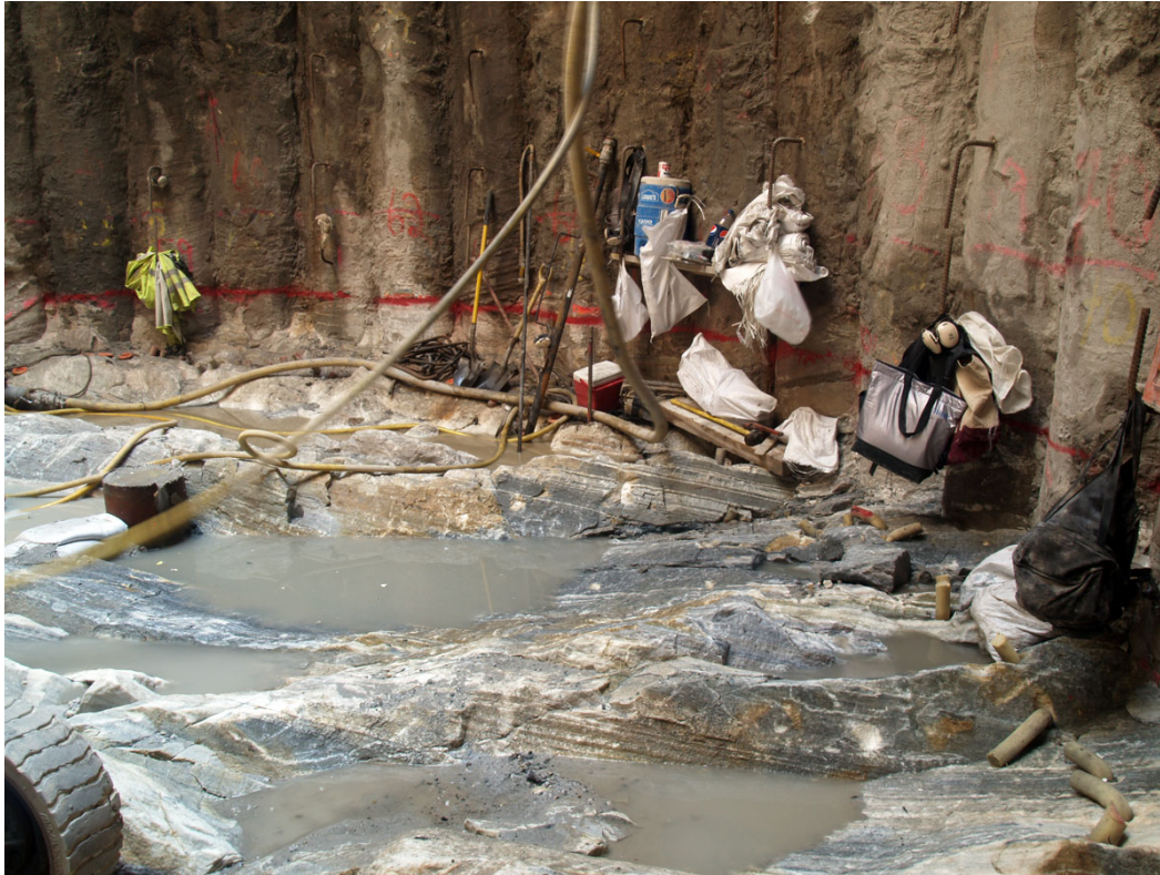
Figure 4 – View of bedrock surface exposed below secant piles about 50' below the ground surface at the Bronx shaft of Con Edison's Harlem River Cable Tunnel. (C. Merguerian digital image taken 03 Aug 2009).
