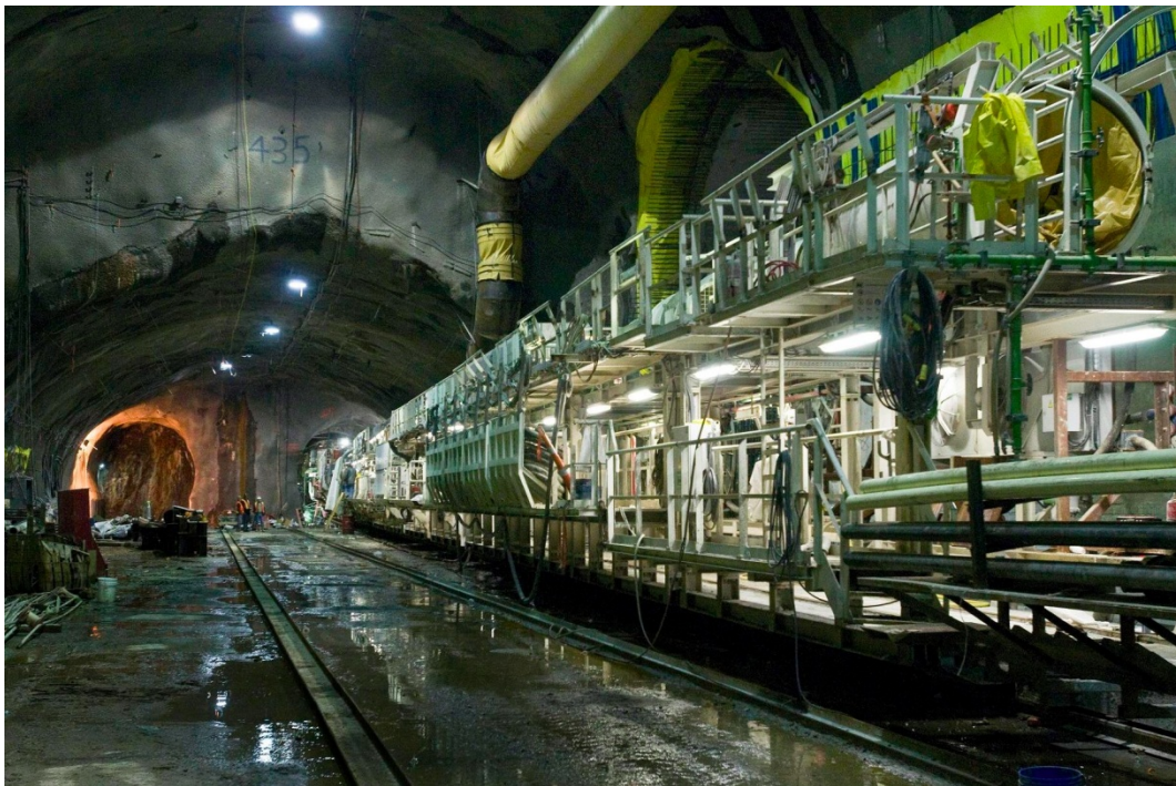
Figure 2 – View N within excavation for the Jacob Javits Convention Center station cavern of the MTA’s #7 Line Extension. To the right note that the hard-rock TBM and trailing gear has begun tunneling. (Web image.)
