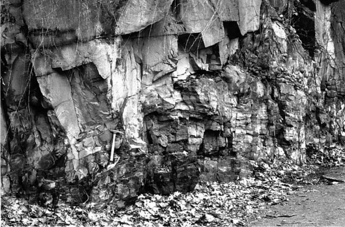
Figure 38. View of a broad E-W-trending arch of the underlying Lockatong in discordant contact with the leading edge of a north-directed ramp. Hammer handle is 40 cm in length and rests immediately above chilled Palisades basalt contact with the Lockatong. (CM photograph).
