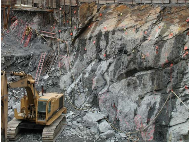
Figure 7 – Condition of west wall (view facing SW) as seen during excavation. Note the multitude of NE-trending faults along the wall that are parallel to the prominent iron-stained fault (#1 from Figure 6). At least five faults were exposed diagonally from the upper right corner of the digital image to the area beneath the church bell tower.
