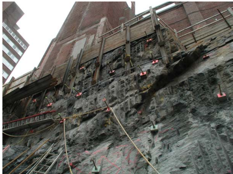
Figure 8 – View beneath the church tower of the “hanging-wall” wedge of Hartland schistose rock above Fault #1 (upper right corner). Note the prevalence of NE-trending faults and joints parallel to the steep iron-stained failure surface of Fault #1 (at least five surfaces visible in this view) and the NW-trending cross fault (Fault #2 in Figure 6) that curves below the wedge.
