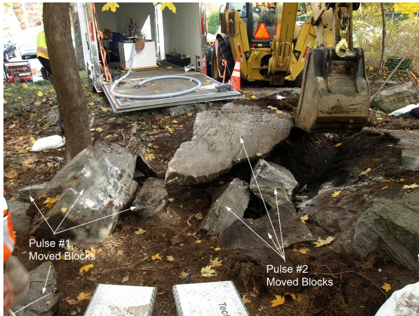
Figure 23 – Largest piece of bedrock (to left of bucket) was peeled from top of exposure after pulse #2. It failed along a steep J_2 joint and a low-angle, weathered J_4 sheeting joint. All of the blocks were readily removed with pry bars and the backhoe. Note the angular, blocky shape of bedrock blocks – failure controlled by main geological weaknesses in rock mass. Rocks removed by the initial pulse were moved by backhoe, beyond this view, to the left of the image. (Dukelabs image taken 17Nov21.)
