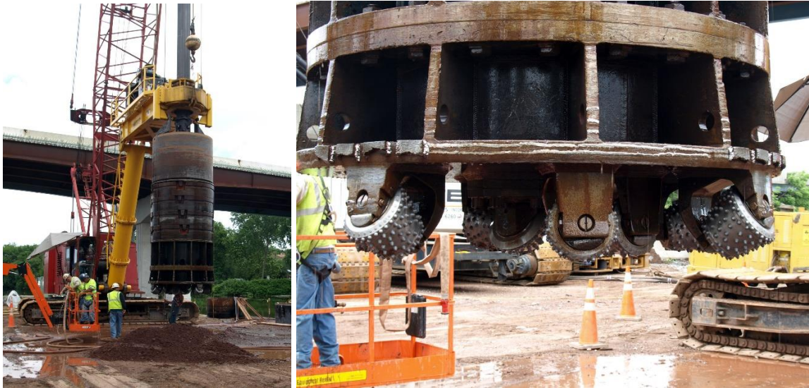
Figure 11 – Westward view of Shaft #23 construction rig near Pier 3 of the job site in New Jersey (L) and close-up view of the cutterhead and cutters (R). (Dukelabs digital images taken 14 June 2013.)
