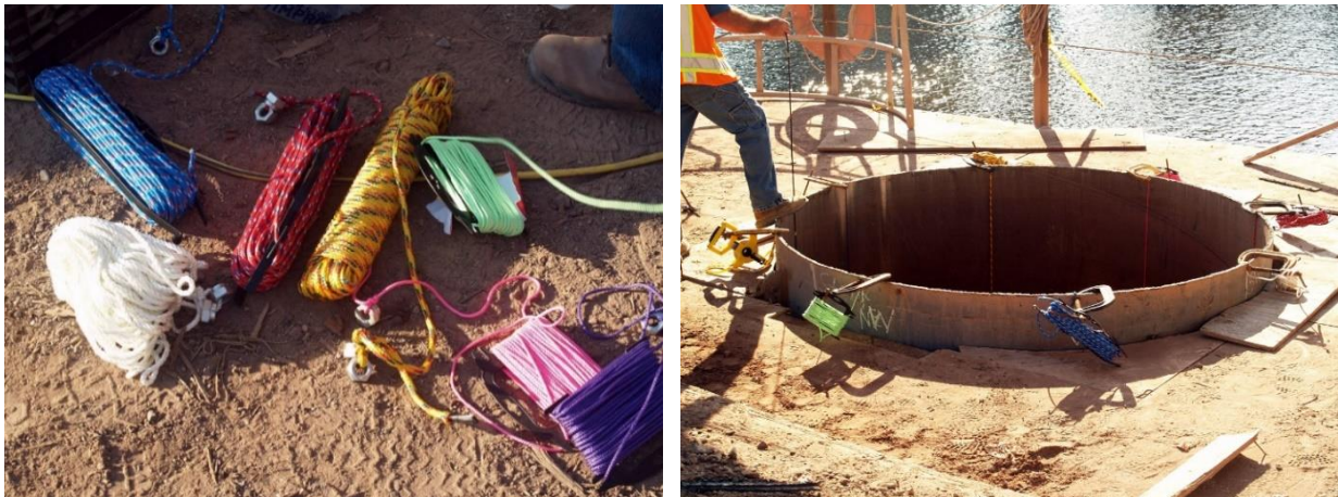
Figure 14 – Various ropes used with weights and C-clamps to hold ropes taught and vertical down the sides of the shaft in order to video each compass rose direction. Analysis of the color-coded videos allowed us to generate an accurate flat 2-D map of the interior of the rock socket.
