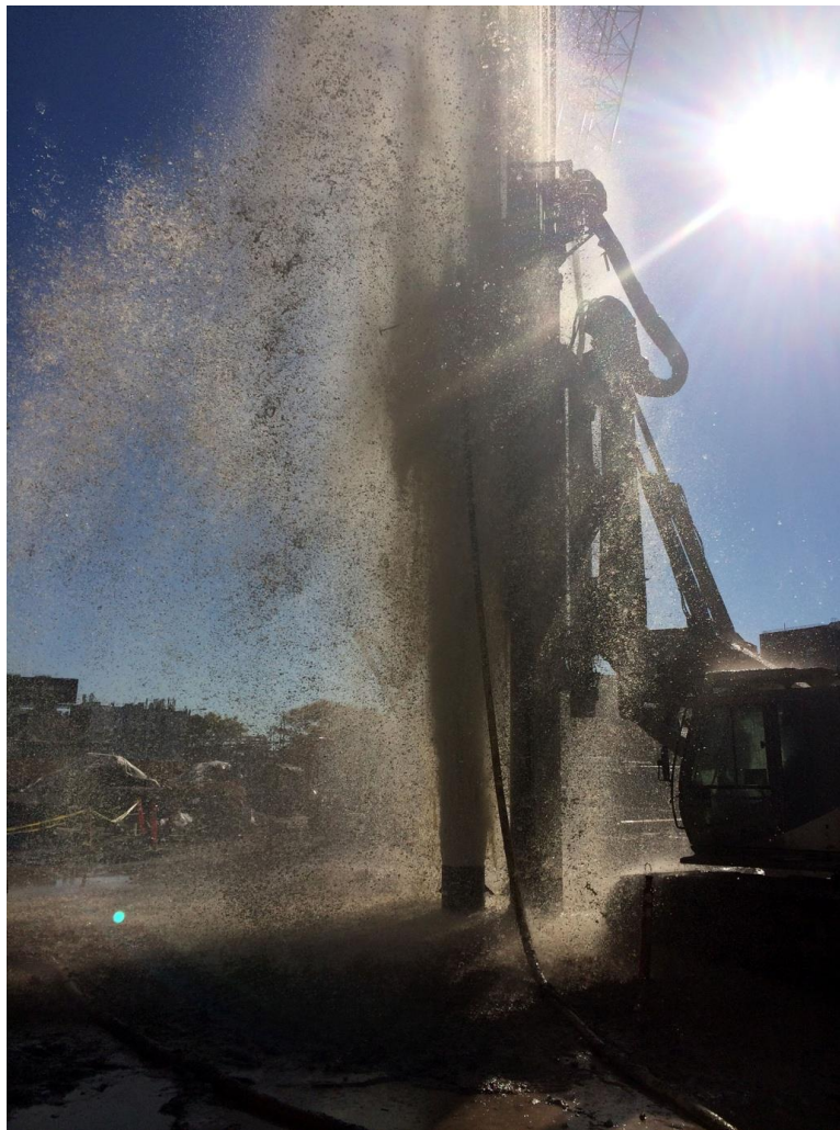
Figure 18 – View of as-built anomalous water + material flow and geysering associated with ~100' deep caisson drilling in November 2015 at the job site. (Contractor image.)
