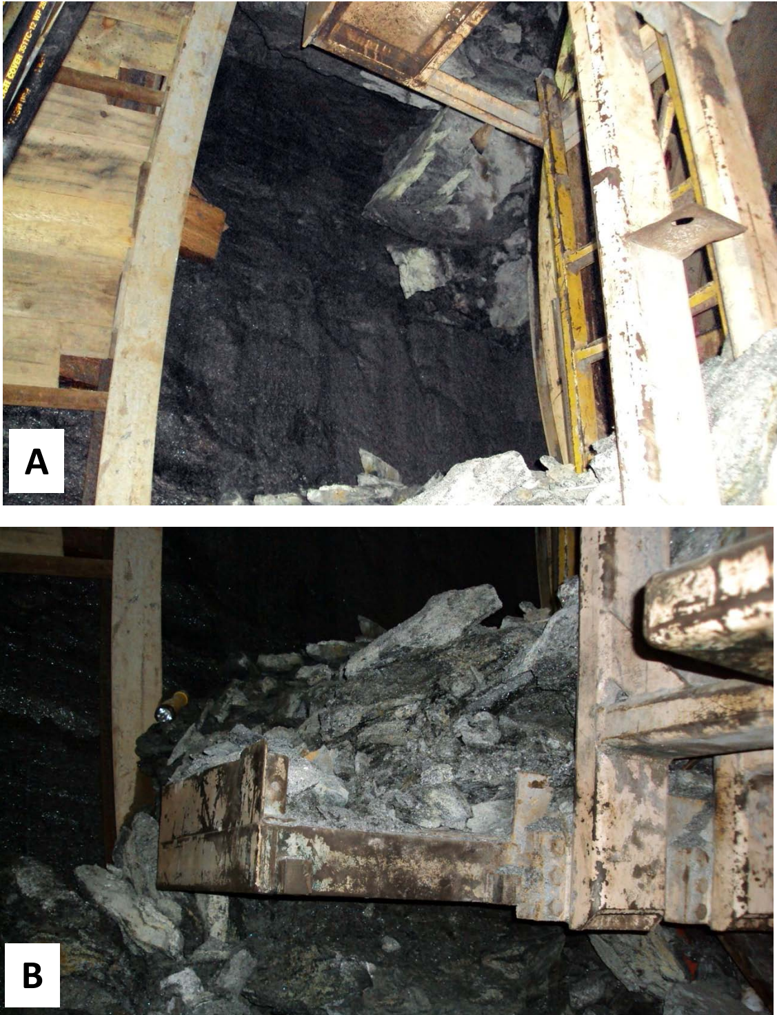
Figure 17. Two views of mucking operations on 09 Dec 2009 showing the extent of poorly-sorted blocky fall out in the left wall rib during mining operations. Upper image (A) shows suspended large blocks. Lower image (B) shows the magnitude of small rocks and weathered clay-rich matrix of fault breccia and gouge associated with the NE-trending fault that traverses the zone. (Progress Photos 28 and 29 provided by Dragados-Judlau JV.)
