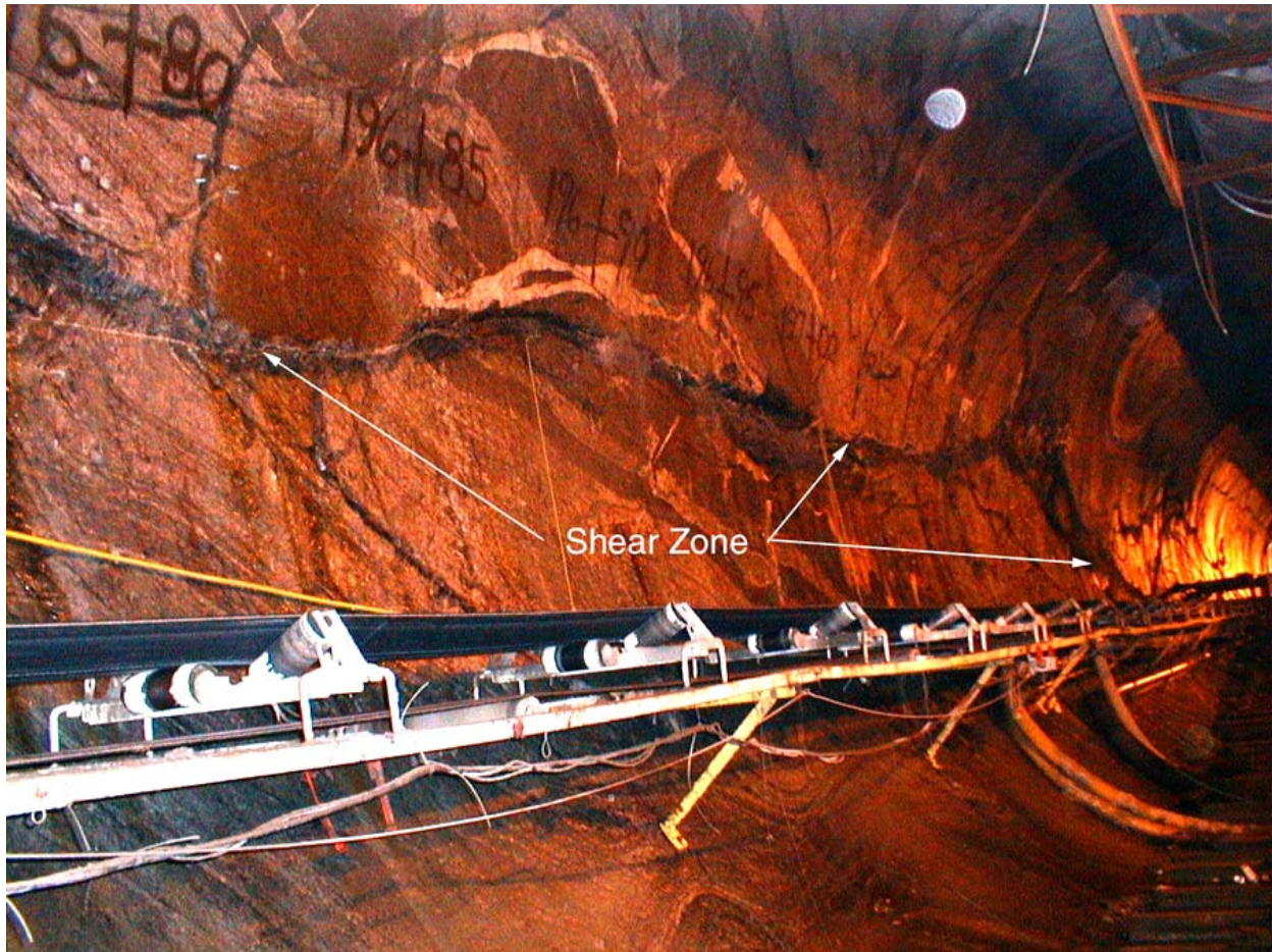
Figure 10. View of migmatitic amphibolite, dioritic gneiss, and minor biotite schist highly fractured because of composite movement along a SW-dipping Group A fault. The fault is a continuous gently dipping feature for 107 m that originates at Station 195+25 and continues on both tunnel walls to Station 198+50. Here it steepens and disappears into the crown of the tunnel in a zone of ramping imbricate fault splays. Fault gouge and -breccia vary in thickness from 0.4 m thick in areas of fault splay intersection near the central reach of the zone to a hairline fracture at the end. (Digital image by C. Merguerian, 18 November 1999.)
