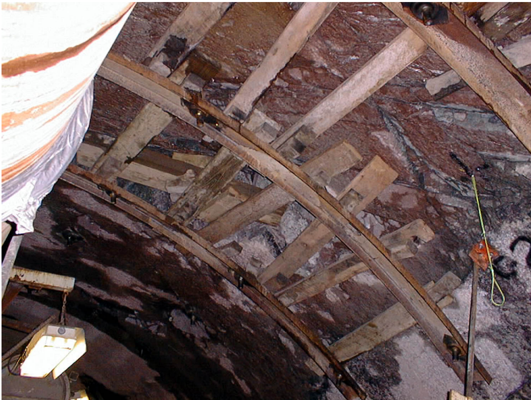
Figure 1 – View of crown and sidewall instability and support in the Queens Water Tunnel, NYC in an area of red-colored rhyodacite dike rocks, unique to the NYC area. The crown failure resulted from internal cooling joints and intersecting NNE-trending faults. Note that the cooling joints cut not only the dike rocks but project into the surrounding gneisses, further extending the area of disturbed ground. The lack of roughness along joint surfaces enabled the blocks to fall freely from the working face, crown, and sidewalls resulting in considerable cutter damage and downtime for repairs and support installation in excess of the patterned rockbolts used throughout the tunnel. (Queens Tunnel station 152+25. Digital image by C. Merguerian taken 27 May 1998.)
