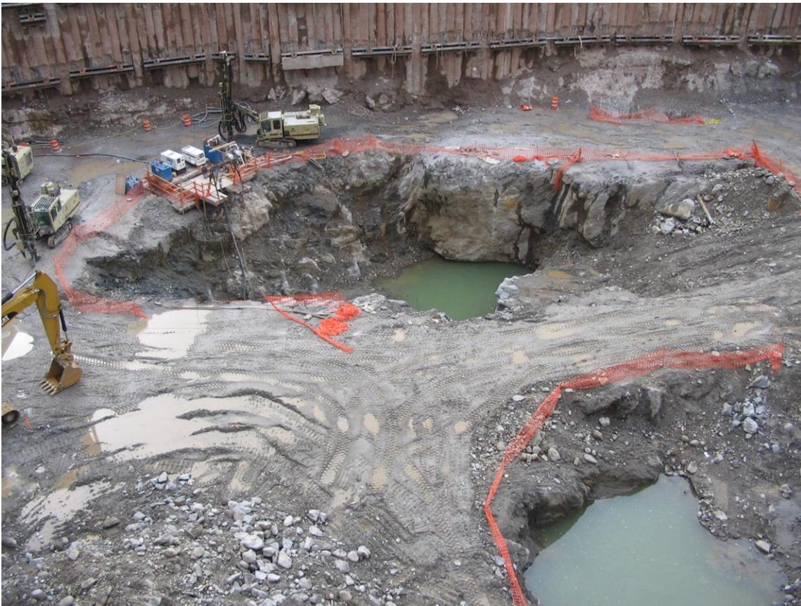
Figure 5 – Two large depressions beneath the Tower 4 site. The western basin (seen at top, facing west) had no outlet. Across the site, bedrock was initially excavated down to El. -60' and the basin bottomed out, under the green pond, at El. -100'. The pond fills a circular whirlpool and plunge pool below a near vertical cliff. During the geotechnical investigation a boring located just behind the cliff face penetrated 11' of pegmatite before entering 32' of till below. A boring on the opposite, eastern side of the basin also penetrated a small ledge of bedrock above till. The eastern depression, lower right corner, was never fully excavated so its true extent is not known. A temporary secant wall keyed into the original top of bedrock is seen along the top of the photo. (Digital image by C. J. Moss.)
