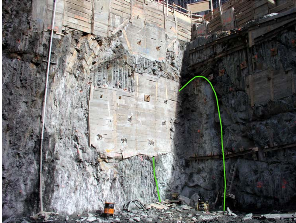
Figure 3 – View of the One Bryant Park serpentinite mass (outlined in green) near the end stage of the excavation showing the surrounding units. By our final visit some of the exposed schistose layers of the serpentinite needed support as they started to unravel along the north wall of the excavation. Support involved the installation of a concrete retaining wall and rock bolts. At this point in the excavation process the overall ellipsoidal shape of the serpentinite mass was clearly visible but the base was not exposed. Digital image taken 07 February 2005.
