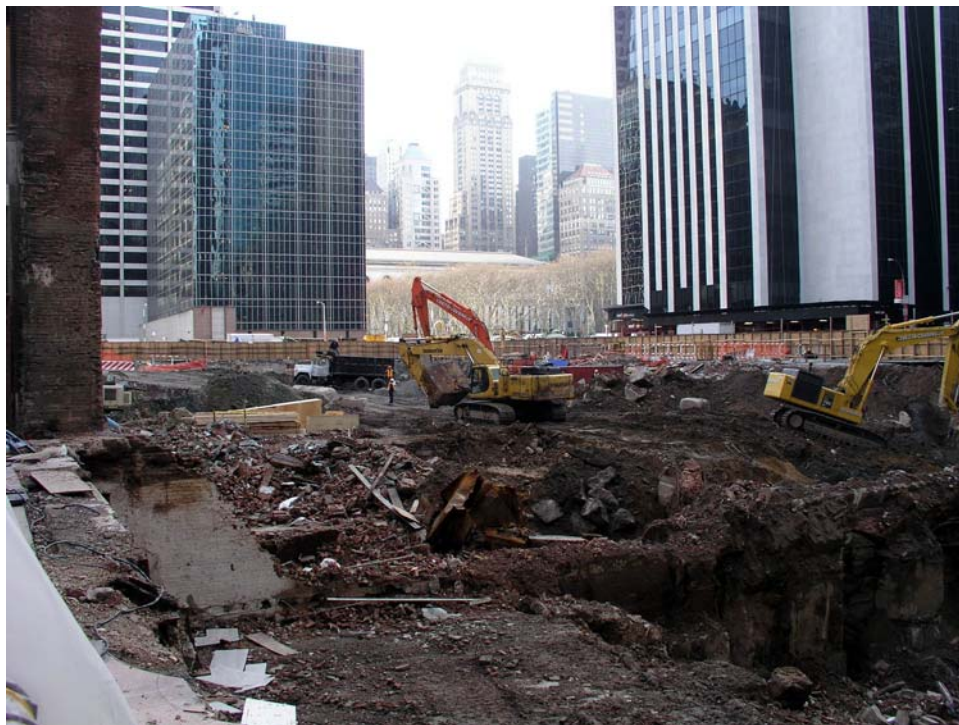
Figure 1 – View toward the SSE (Bryant Park in distance) of the One Bryant Park site showing the early stages of the excavation. Digital image taken 21 December 2004.
